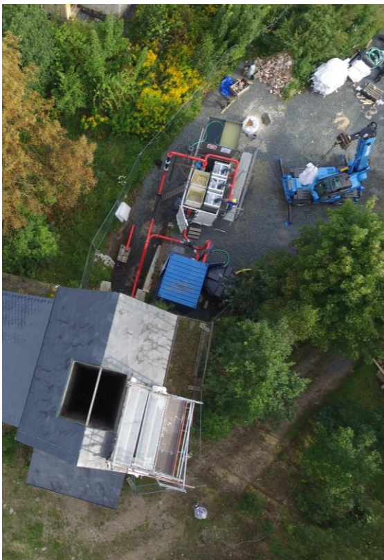
Figure 1 Top-view of above-ground construction. Riser and fall pipe are located just below roof hole, see next figure. Source: Lutz Weidler
